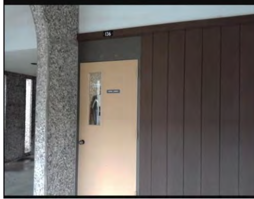
Should have signage next to door with brail
