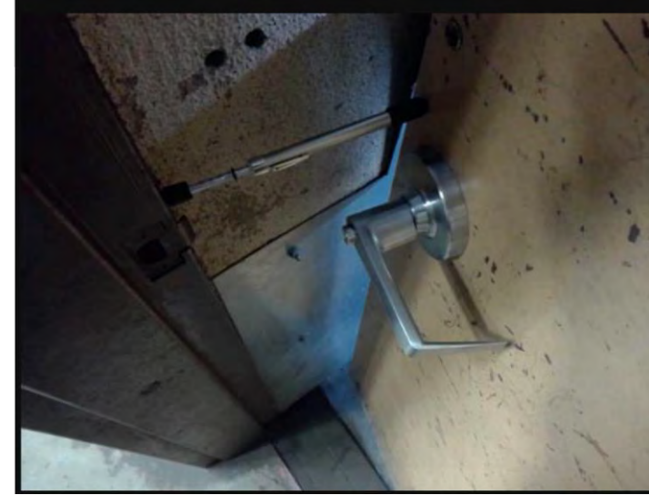
Door closing pressure too high
