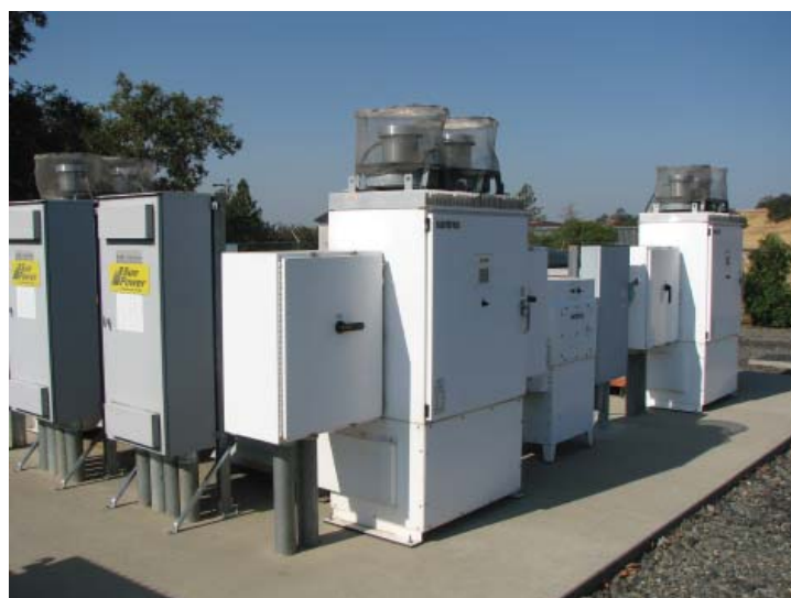
Phase I solar inverters
