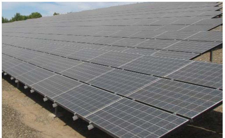
Solar panel array
