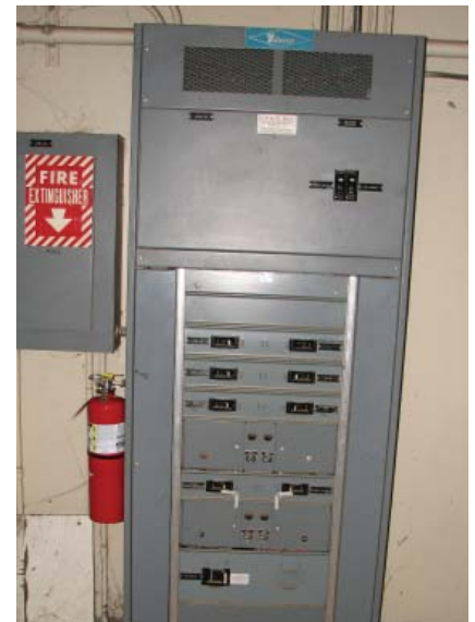
Original electrical panel
