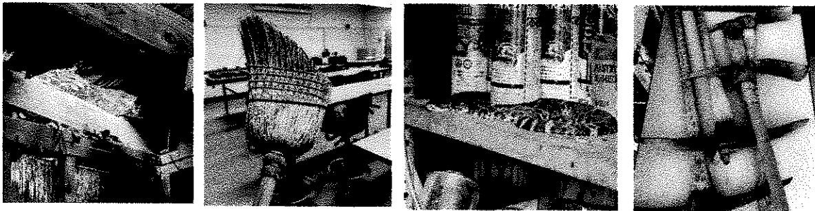
ABOVE: Current equipment storage repairs needed, failing or unsafe equipment and wildlife entry from holes in equipment storage area.
