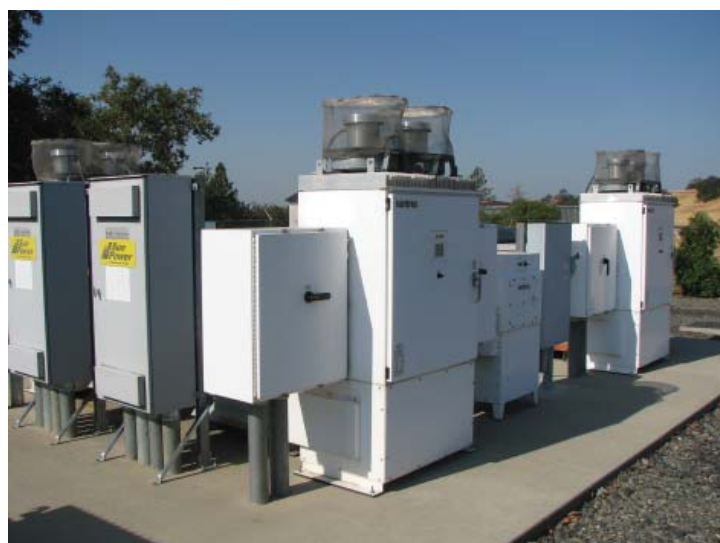
Phase I solar inverters
