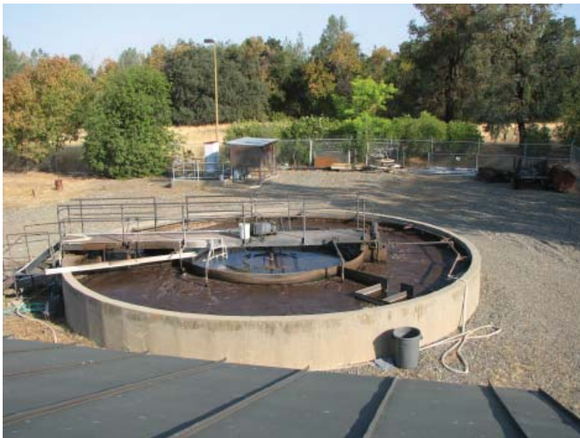
Sewer treatment plant
